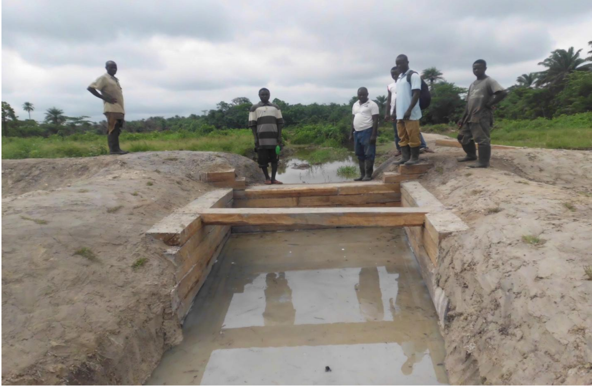
View of the completed spillway in Kpodo Swamp, Zayglay Town, Nimba County, Liberia.
